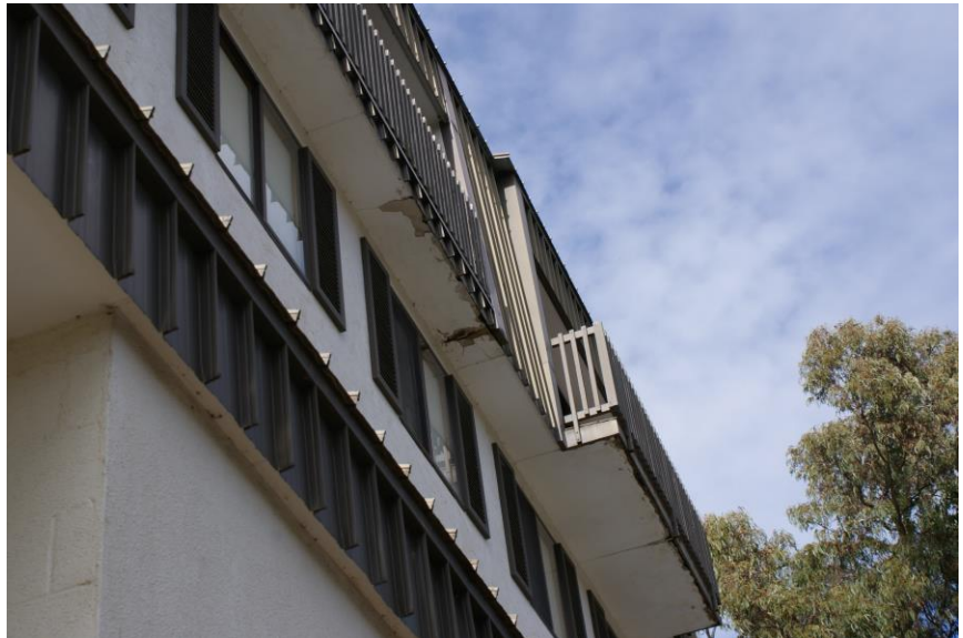
Figure 7 : Photo of the northern elevation and Juliet balconies to be replaced with the larger deck/balcony
