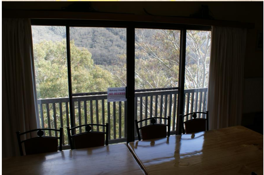
Figure 6 : Photo of the existing Juliet Balconies to be replaced with a larger deck/balcony
