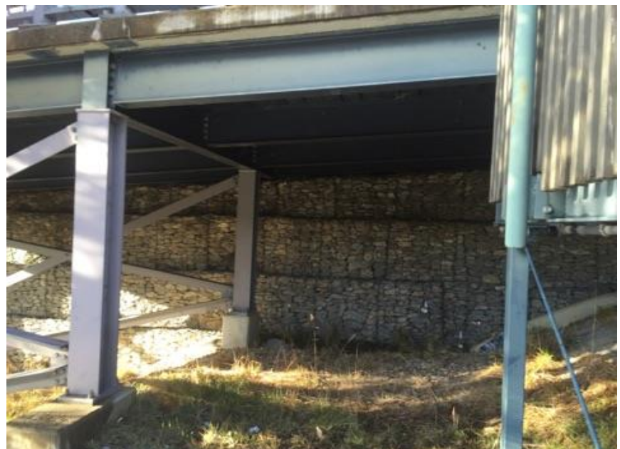
Figure 12: Photo of the car park undercroft area to be used for the installation of a bike store cage
